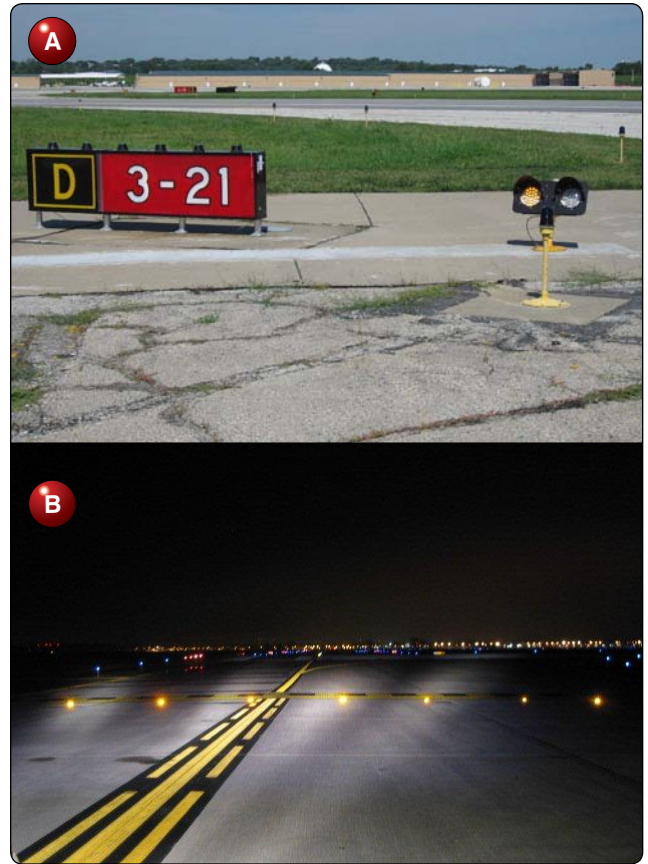
Figure 1-26. (A) Elevated flashing yellow runway guard lights also referred to as “wig-wag” lights. (B) In-pavement flashing yellow runway guard lights.
